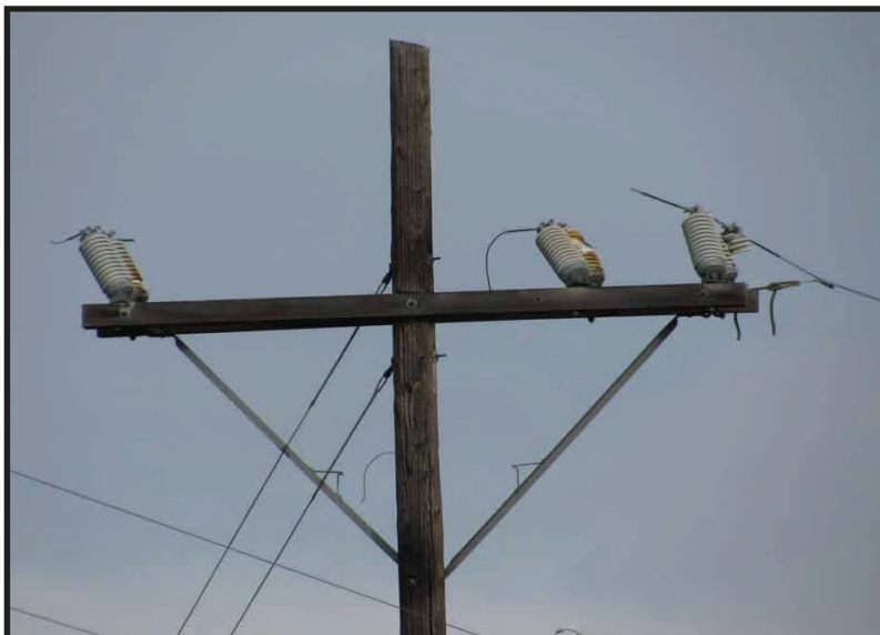
NorthWestern Energy transmission line showing the broken and burnt insulators located south of the Three Mile Fire Station.
