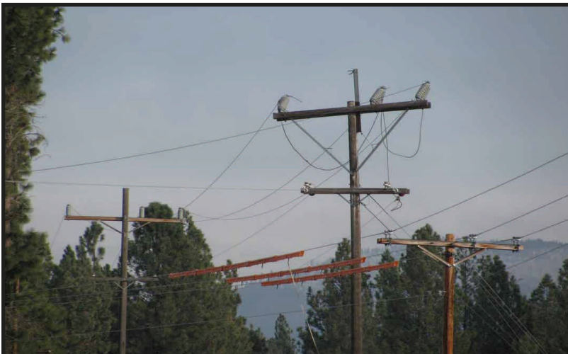
NorthWestern Energy transmission line south of the Three-Mile Fire Station on Eastside Highway showing the downed wires.
